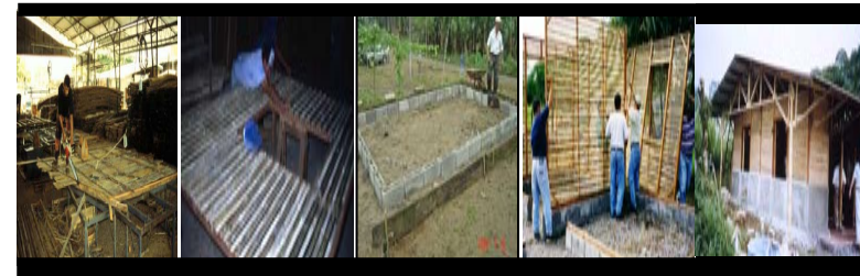
Figure 5. Production of and Building with Innovative Prefab Bamboo Construction Technology. Source: Janssen, 2000 (personal collection).
