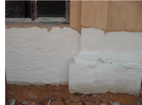
Figure 2. Treatment of Salt Desalination on Wall Surfaces Through the Process of Poulticing
